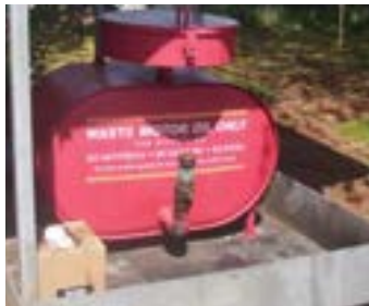
Waste oil tank at Tomahawk Bay Marina
